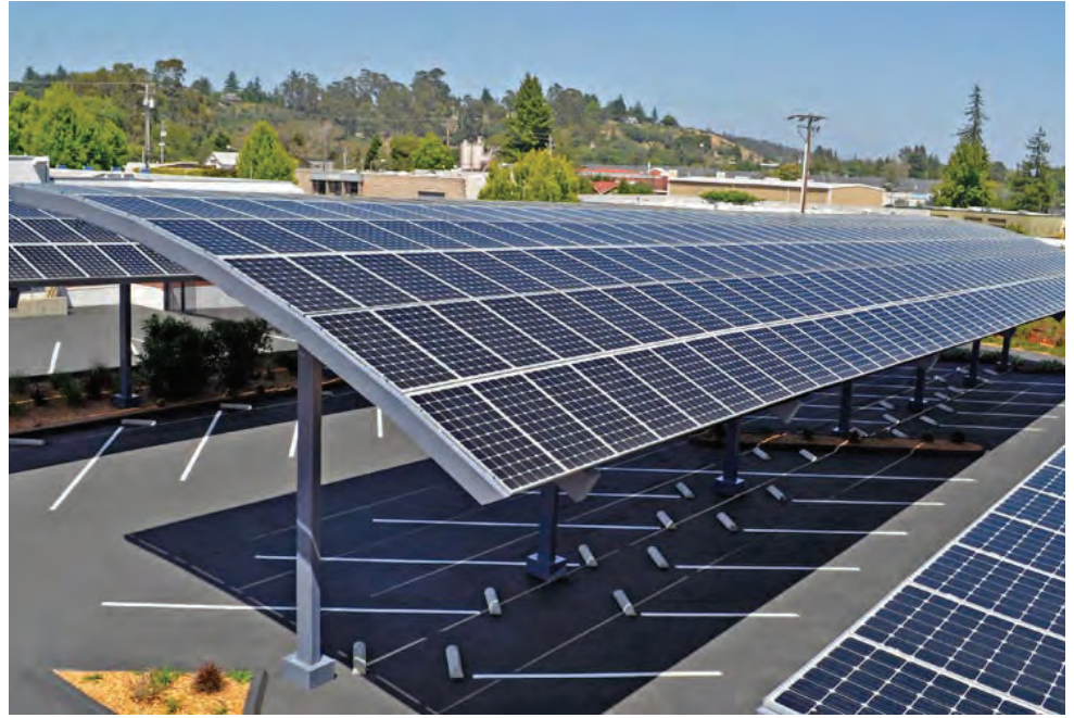
Land use can be optimized by installing photovoltaic shading structures on large surface lots to provide a source of renewable energy, mitigate the impact of heat island effect, and provide shade for humans and vehicles (Solar City JS Beam Carport Parking Structure)
