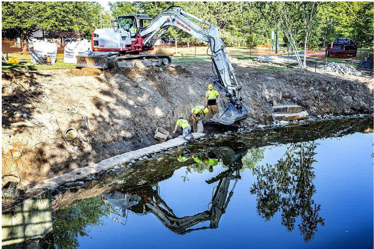
A crew is currently working on the stream outlet near Alumni Plaza. The project is intended to stabilize the bank of the St. Joseph River to prevent erosion, while looking attractive.
