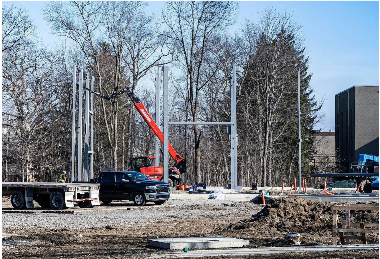
Construction activity on PFW's new Surack-Sweetwater Music Industry Building is trending upward.
